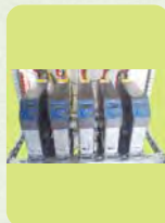
inside view of capacitor panel
